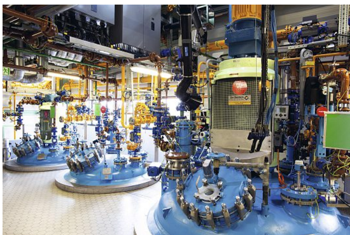
Fig. 3. Multipurpose production reactors at DOTTIKON (Credit: Anja Wille/DES).
