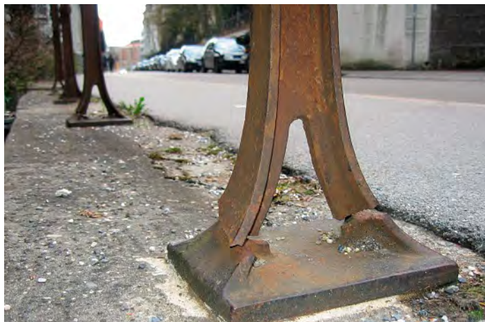
Corrosion is an economic issue since it destroys material goods
